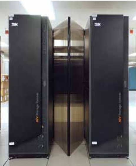
Single Unit Installed between a row of racks.
