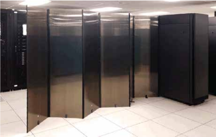
Multiple units coupled together to create barrier wall with a rack row.
